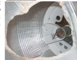
Ruptured Type-S Lamp that melted through a plastic lens
